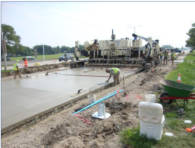
Crews paving the southeast quadrant of E. Layton Ave. and S. Howell Ave.
