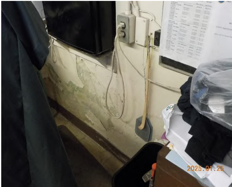
[Engineer's Office] Room 003 – West wall B deterioration (cracking/peeling paint)
