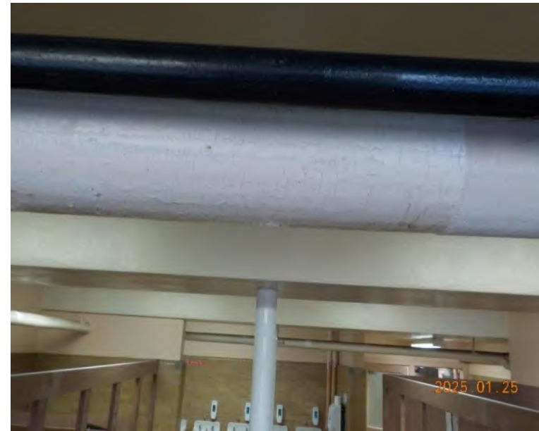
009 – system pipe by windows along outer wall C (cracking)
