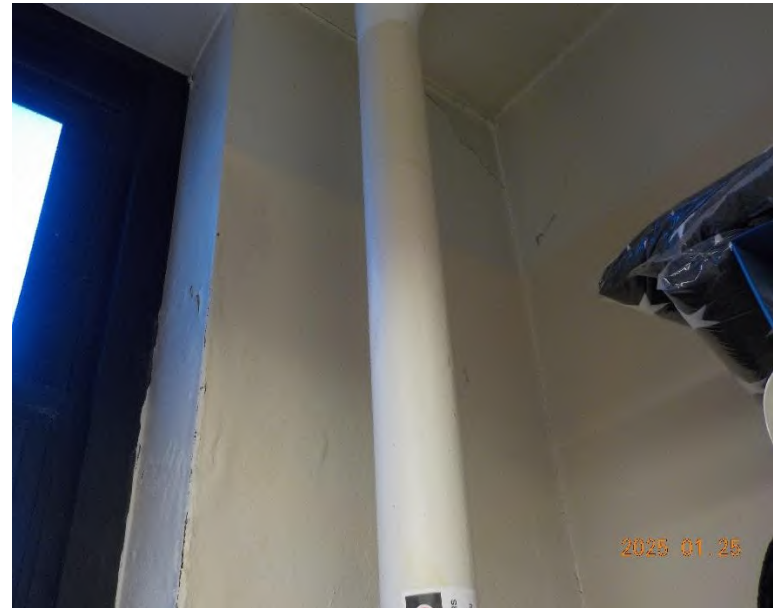
Rm 003 North wall C (cracking/chipping)
