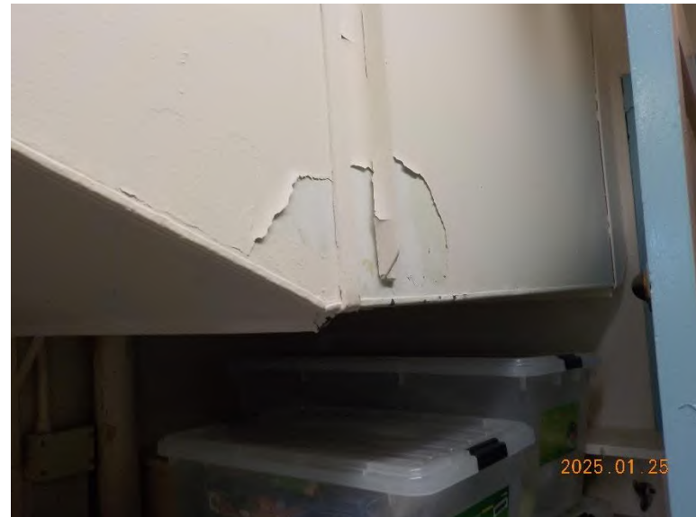
Rm 008A – HVAC duct wall B - deterioration (peeling/pickable)
