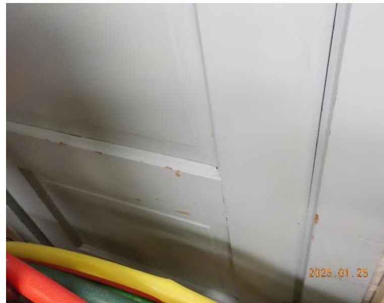
Rm 006A – door-trim & door to Rm 006 (chipped paint by hula-hoop storage)
