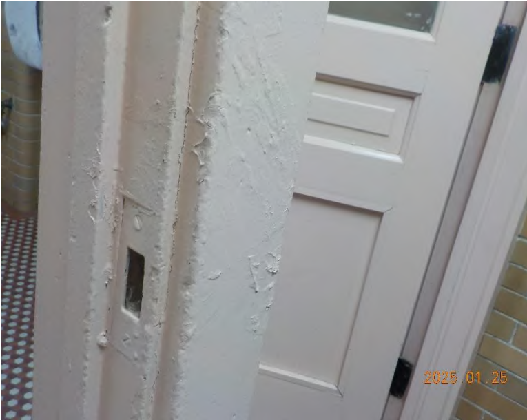
Boy's bathroom 002 door trim/jamb (pickable paint)
