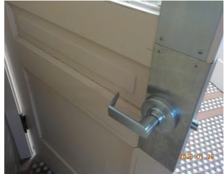
Bathroom 002 entrance doors show cracked/pickable paint along door panels, both sides of both doors
