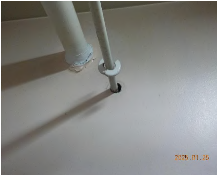
009 – East wall D – (cracked/chipped paint around pipes)
