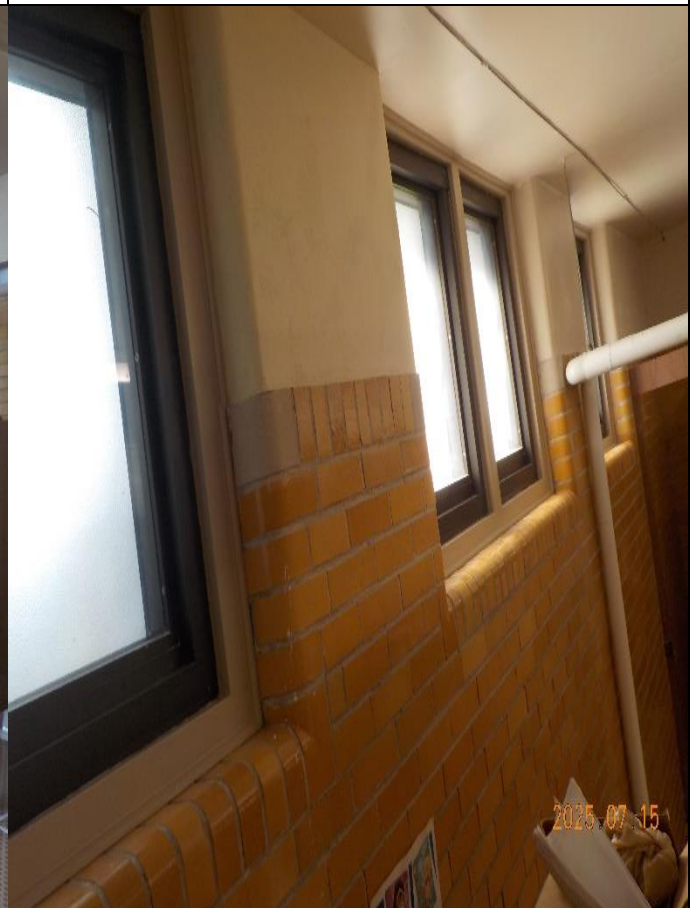
Girls' Toilet (001) windowsills (indicative of Boys' Toilet condition)
