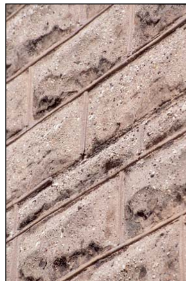
The Kren Building features molded concrete block with half-round, convex mortar joints.
