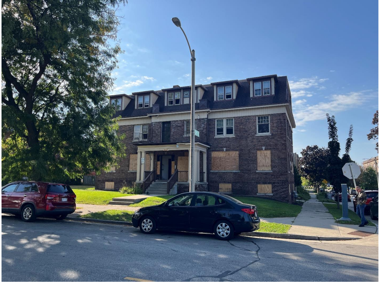
Figure 6. 3131 West Wells Street following the July 2025 fire.
