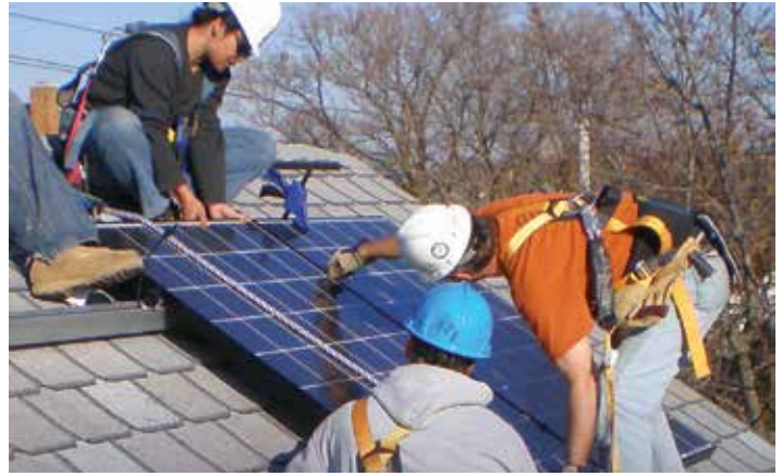
Rooftop solar installation. Photo Credit: MREA
