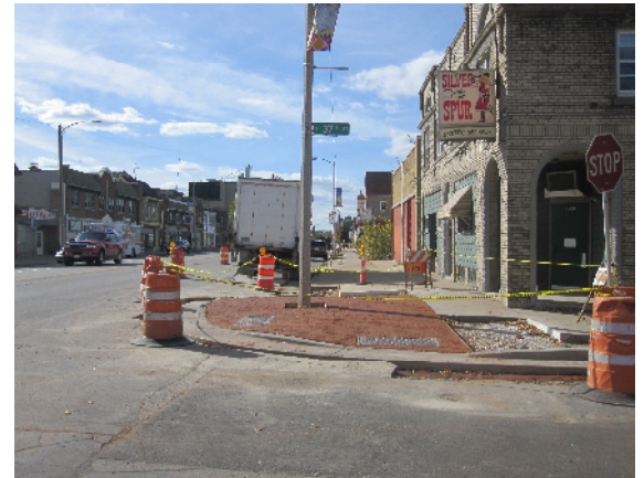
Above: Work in progress at S. 37th including curb push-out and terra cotta colored and stamped concrete with pedestrian ramp.
