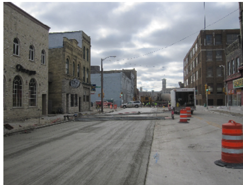
View looking south on 2nd Street as crews work to complete concrete installation
