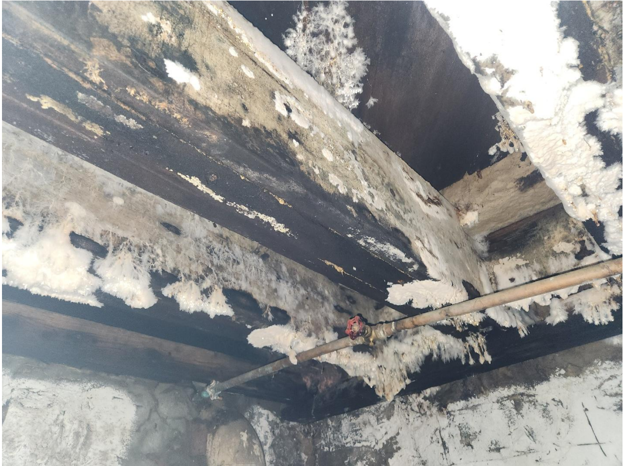
Basement Fungal Growth
