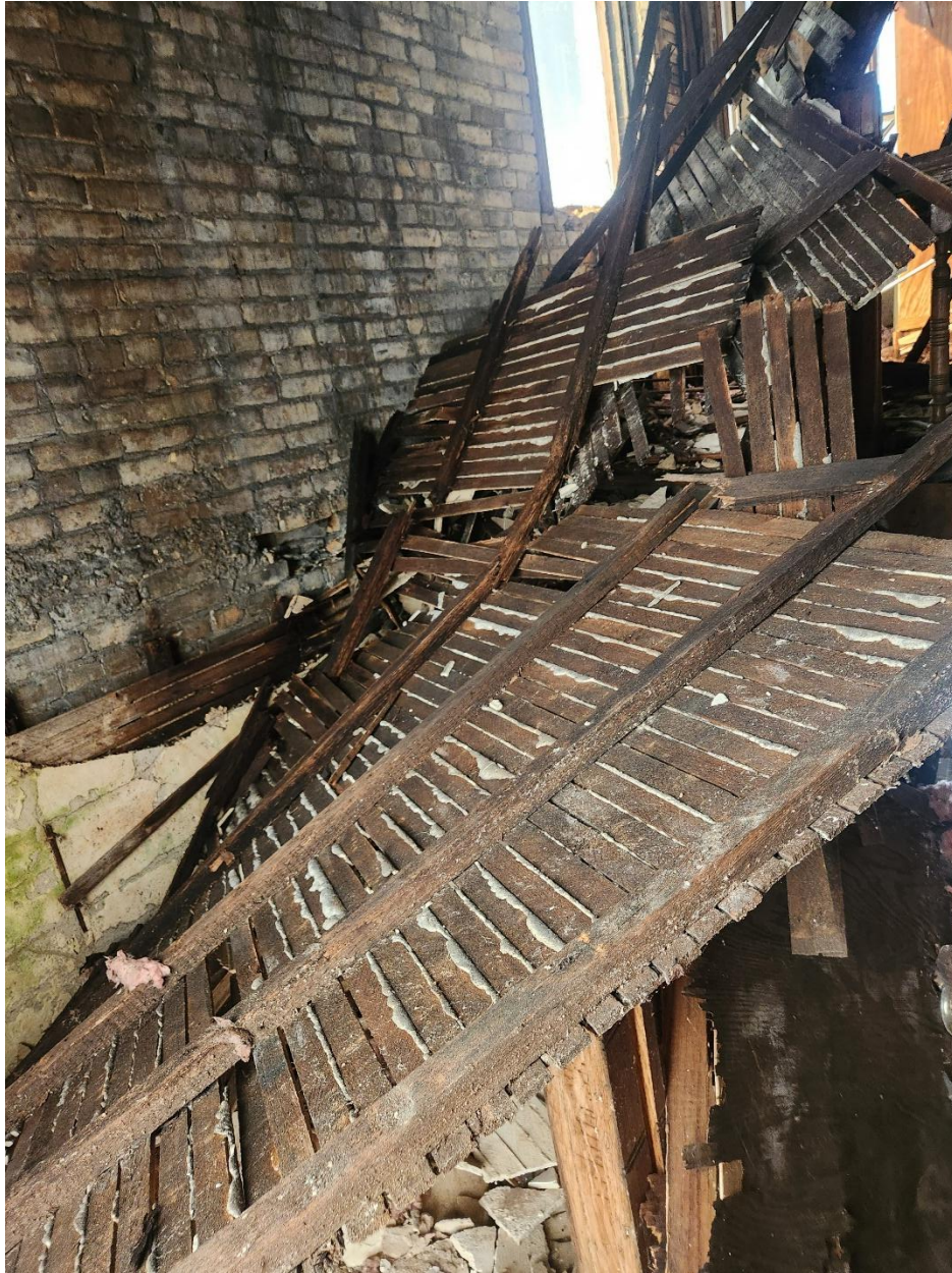
3 rd Floor Stairwell Plaster Wall Collapse
