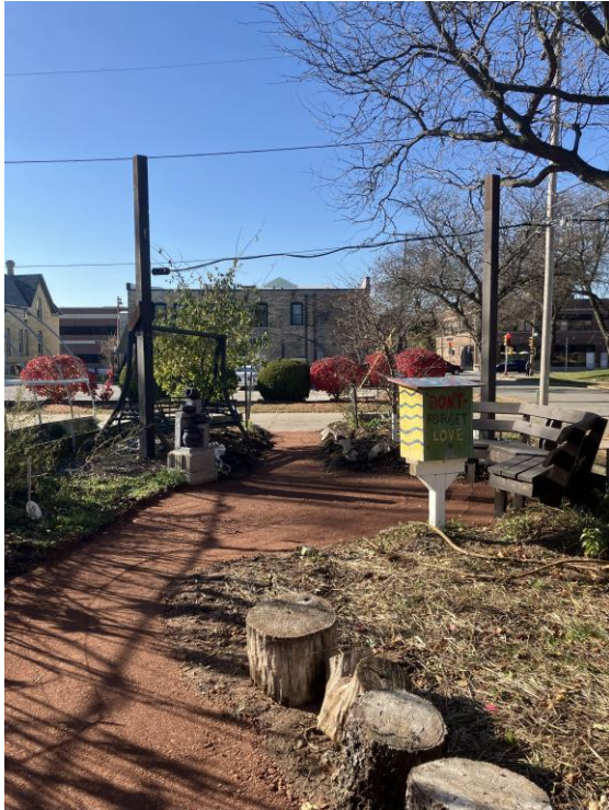
The results of the new pathways installed at the Breathing Spaces, including opening the space for accessible entrance from both sides.
