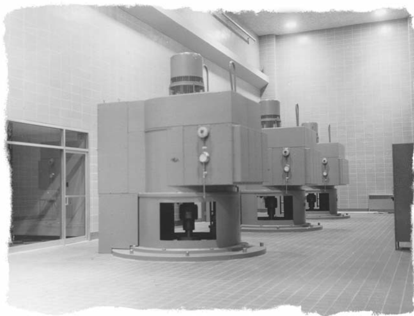
New pumps at North Point Station, 1964.
