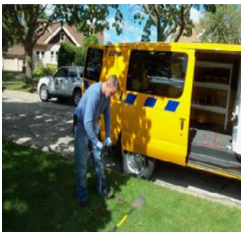
A Meter Services Technician opens a curb stop that allows water to flow from the water main in the street through the homeowner's lateral pipe to the house.
