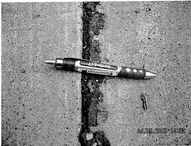
Photo of faulting
