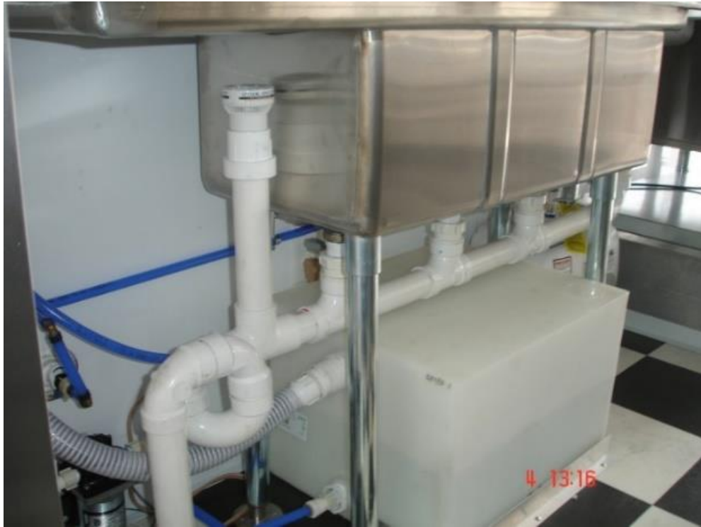
Example of a "clear" water tank where water is visible
