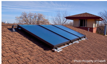
Solar Hot Water at Engine House #23
