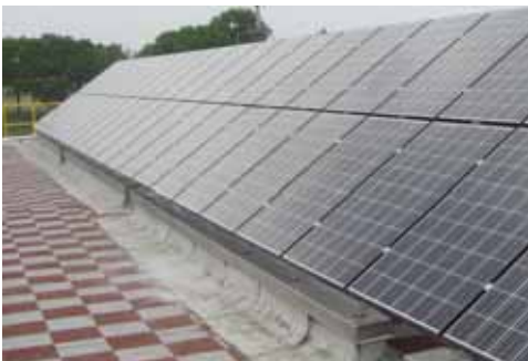
Photovoltaic Panels Cooper School - Milwaukee, Wisconsin
